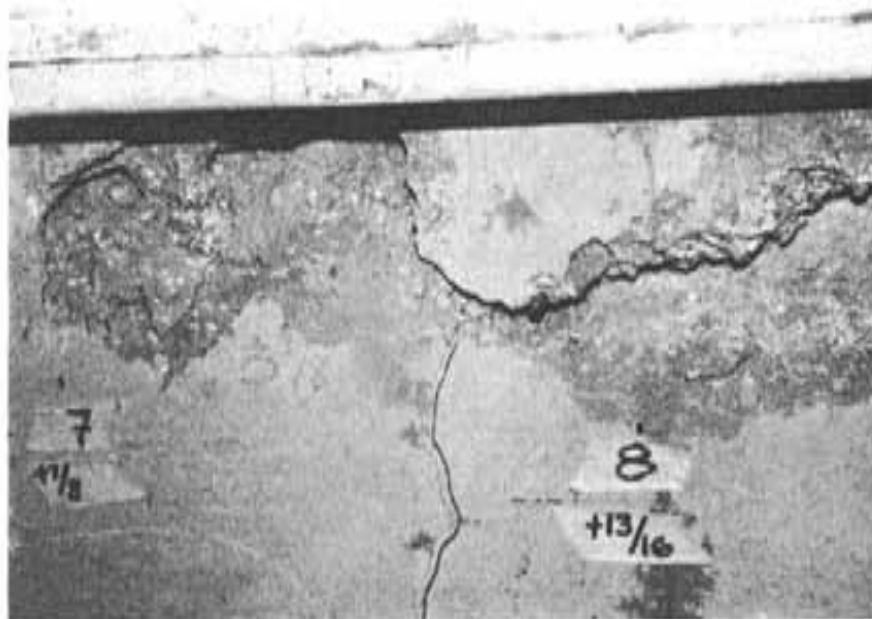
Figure 2.3 Shotcrete wall separations and voids
